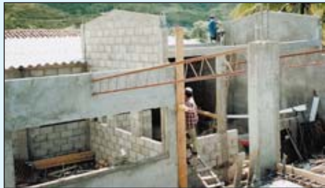
The nutrition center seen here under construction was the idea of the Dethlefses’. The center was completed last June.
