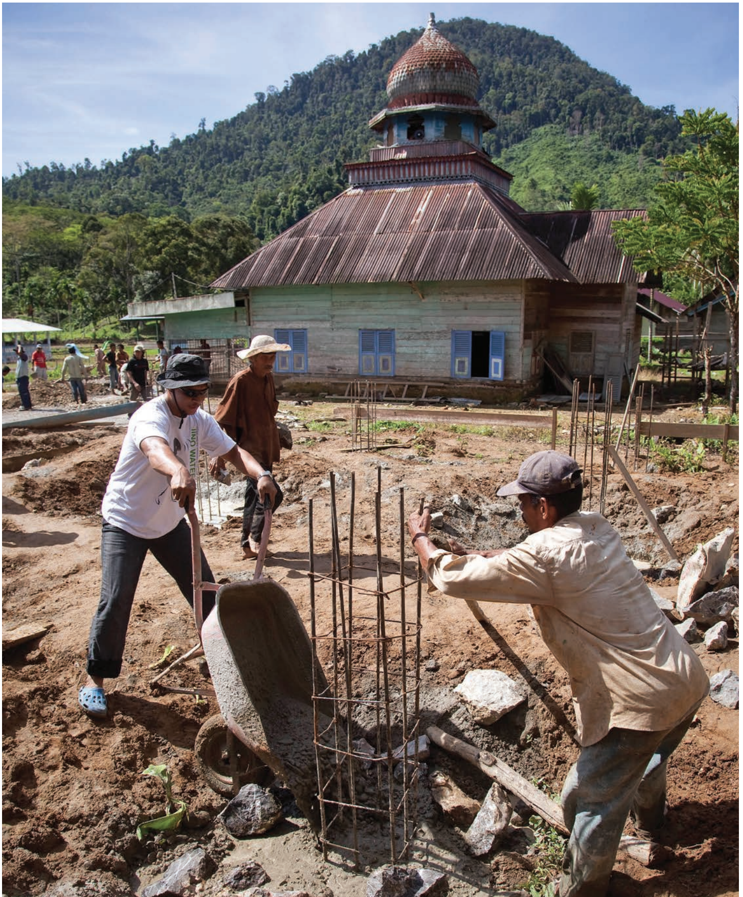
In the village of Lawe Buluh Didi (population 250), JRS project coordinator Donatus Akur, left, assists villagers in pouring the foundation for a mosque. It took a year and a half of negotiations for the community and JRS to achieve an agreement to work together on the project. The community supplied the labor and JRS helped fund the effort, about $25,000. Fr. Doll notes that a mosque is more than a place of worship here; it is the community's gathering space.
