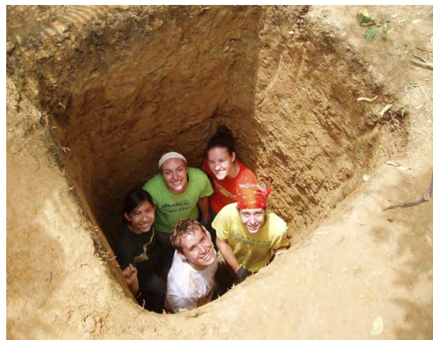
Participants standing in a hole that they just finished digging. This hole will be used for a newly constructed latrine for a family. The latrine will provide a central location for human waste, benefiting the health of the family and entire community.
