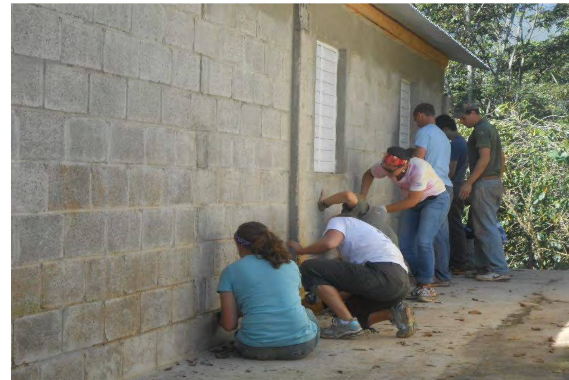
Participants work to sand the outer wall of a new community clinic in the campo of Las Lagunas. The closest clinic, other than this facility, is hours away. This clinic is now fully functional and serves as a health resource for the community.
