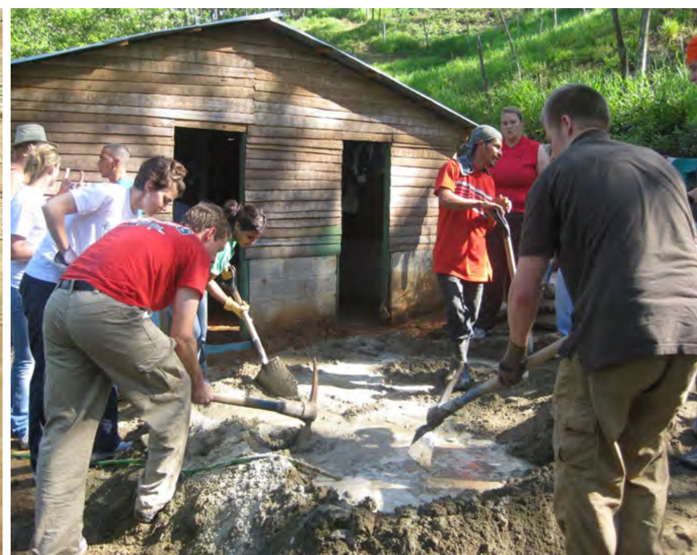
Participants laying concrete that will replace a dirt floor in a family's home. This provides the family with a sanitary and permanent living space and the opportunity for a more healthy lifestyle.
